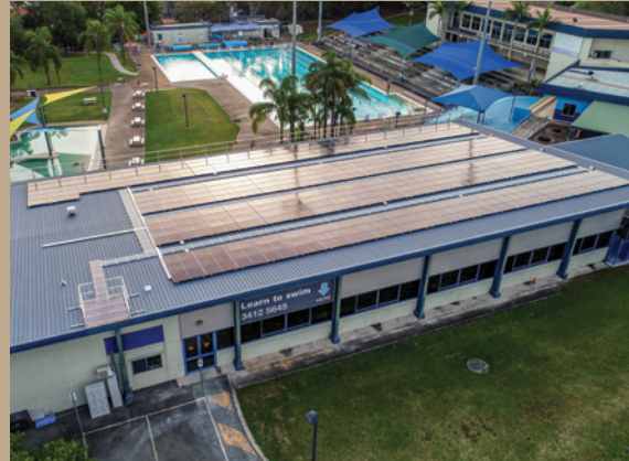
Solar PV panels on Logan North Aquatic Centre Roof top
