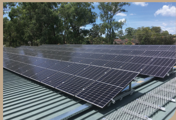
Solar PV panels on Marsden Library Roof Top
