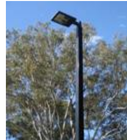
Figure 4 – Photo displaying light and pole
