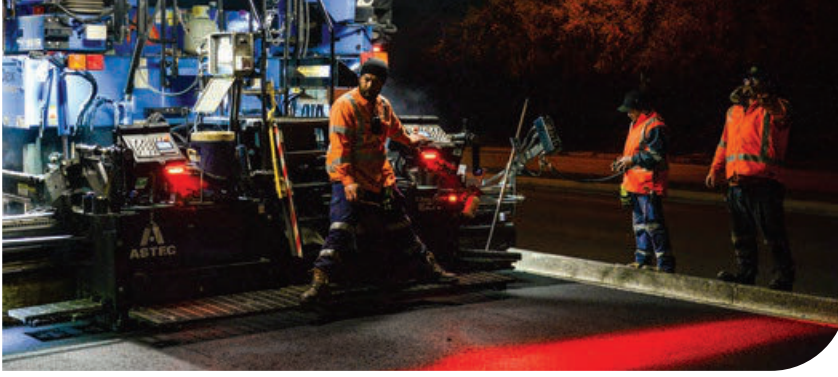
Council road crews working at night to help avoid disruption to daytime traffic.
