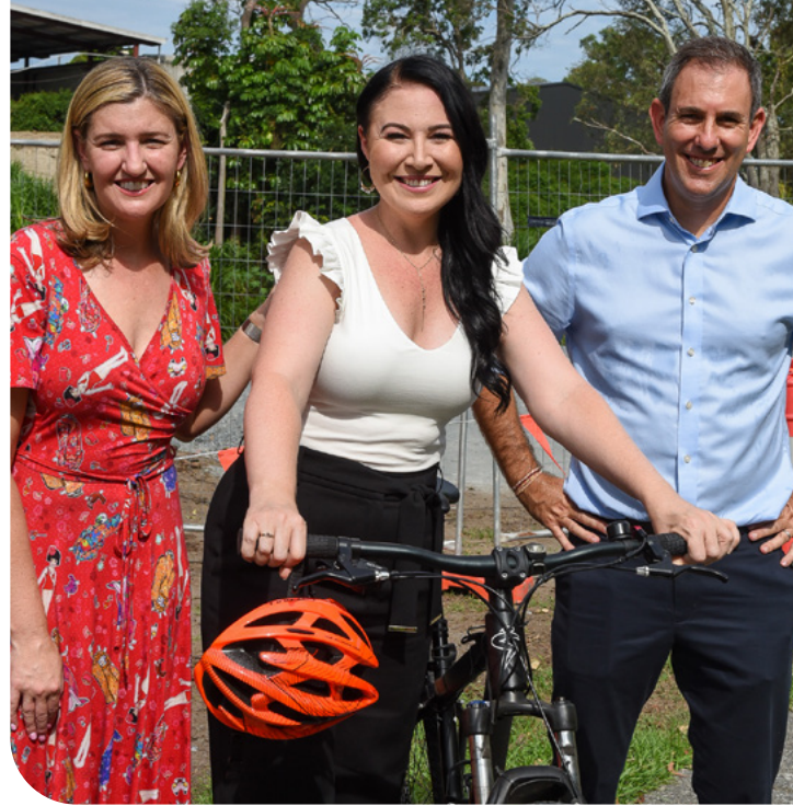
Councillor Mindy Russell (centre) with Federal Treasurer and Member for Rankin Jim Chalmers and Queensland Attorney General and Member for Waterford Shannon Fentiman, at the construction site of the Slacks Creek Shared Path extension.
