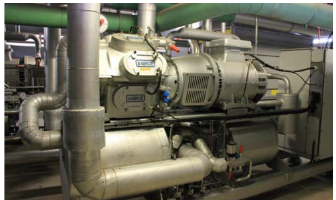
Ammonia chiller at the Council Administration Centre
