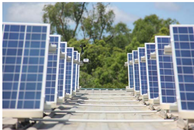
30 kW solar PV system at the Logan Recycling Market
