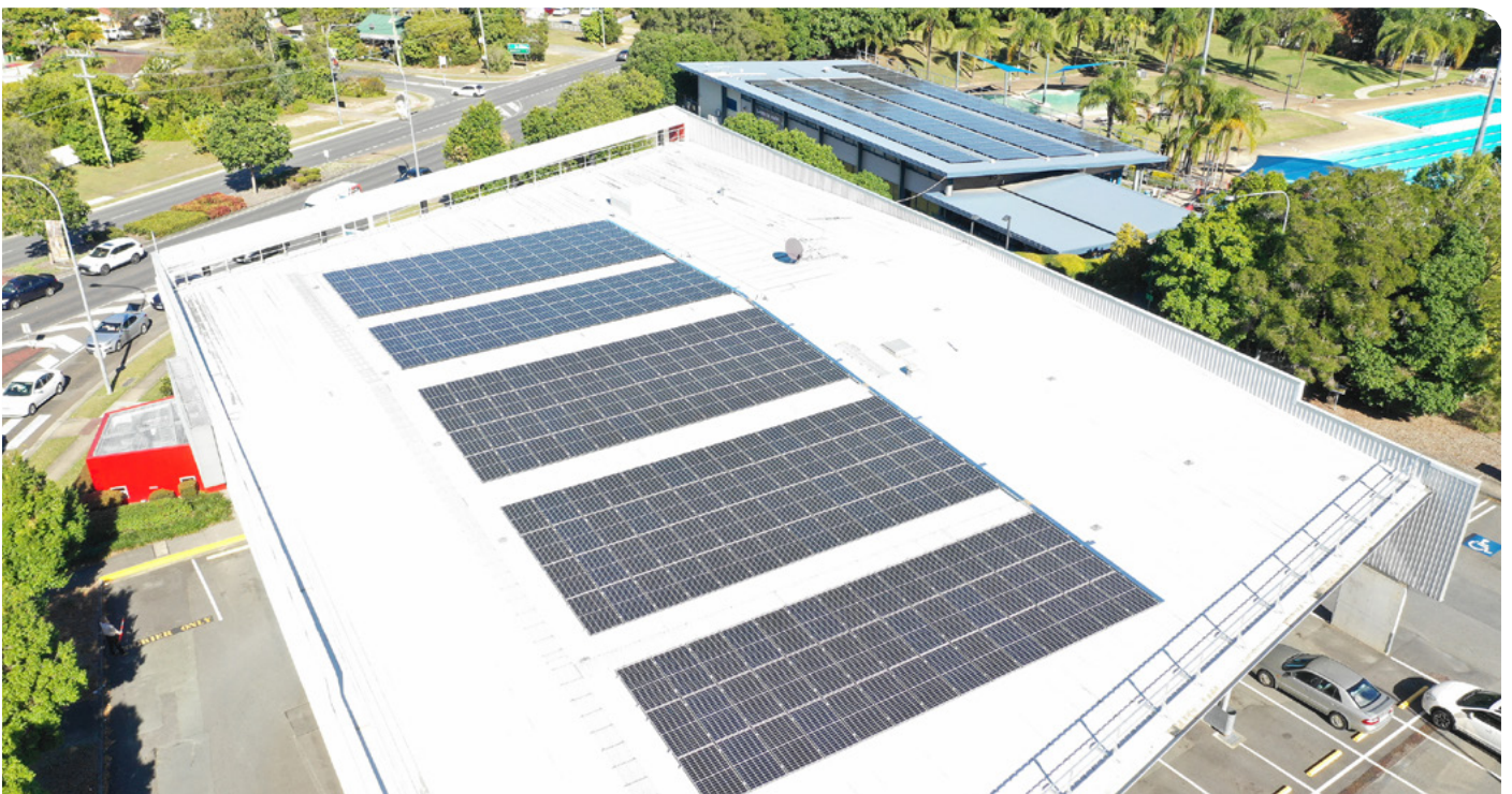
Solar panels are helping to power Logan North Library (foreground) and the Logan North Aquatic Centre (background).
