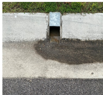
Approved outlet to Council's stormwater drainage system.
